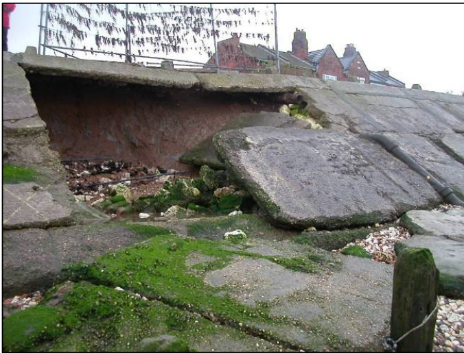
Photos 1 & 2 showing deterioration of the existing defences in the Humber at 1) Paull Village on the north bank and 2) Immingham on the south bank
